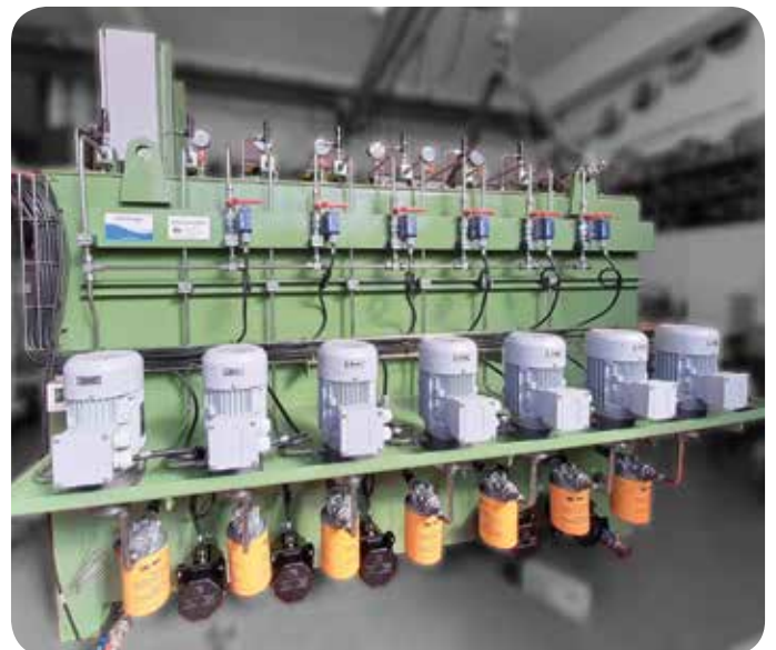
OIL RECIRCULATION SYSTEMS
